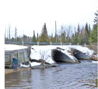
RiverProjectMtgPhoto; The current double 16' wide culverts that sit where Old State Road crosses the Jordan River are slated for removal this spring. COURTESY PHOTO
